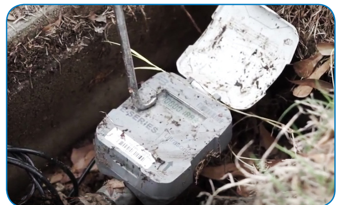
E-Series Ultrasonic Meter in pit application.
